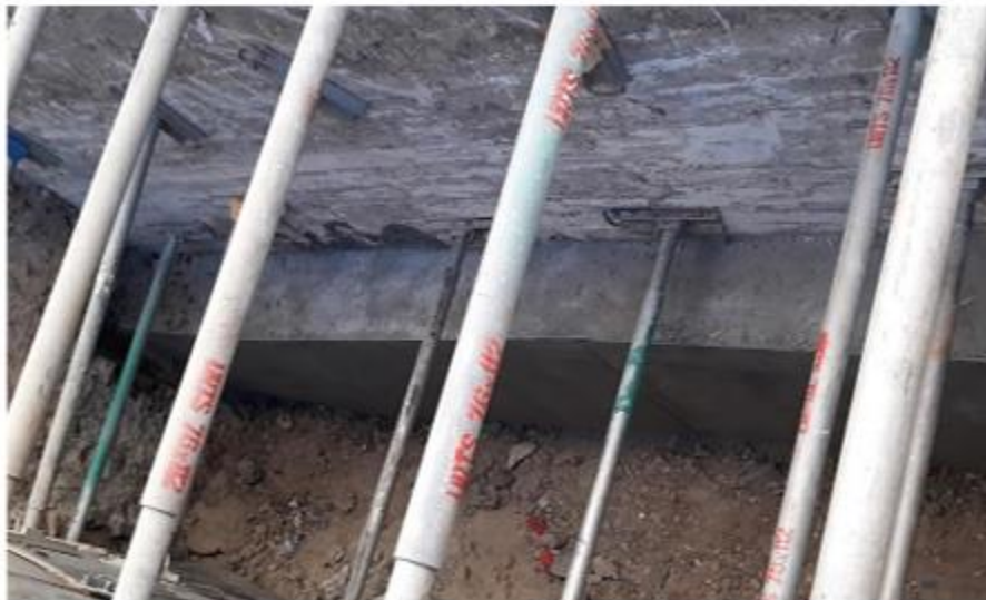
Concrete Underpinning Reinforcement for the Foundation of the Main Building Source: AP Construction
