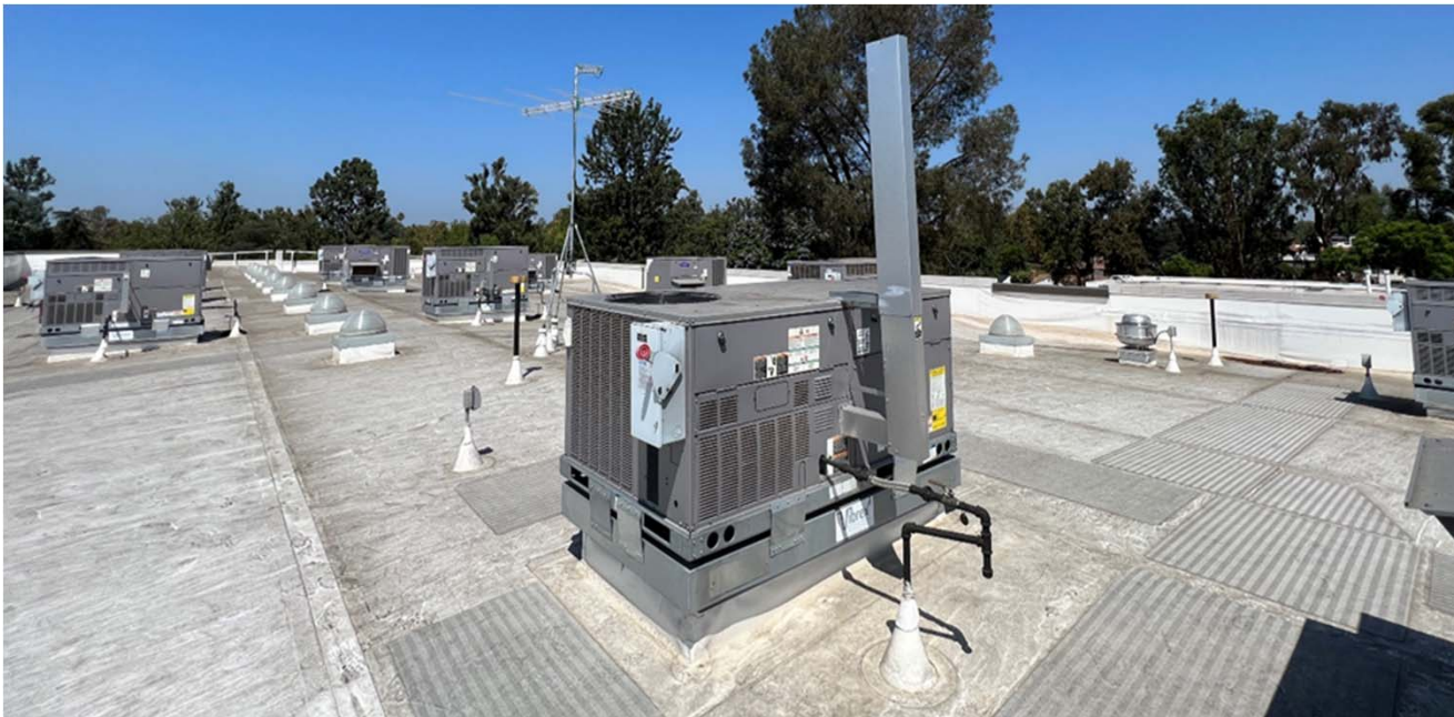
Colfax Charter ES Main Classroom – HVAC Roof Top Units (OIG Photo – 10/12/2022)
