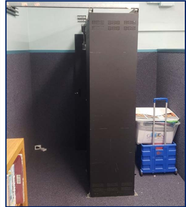
Public Address (PA) System to Remove
