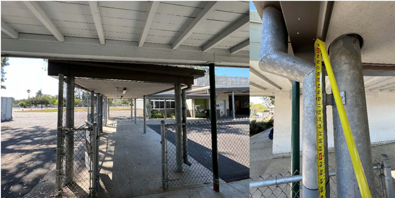
Kindergarten Walkway Canopy – View of Entry and Canopy Height Measurement (OIG Photo – 9/6/2022)
