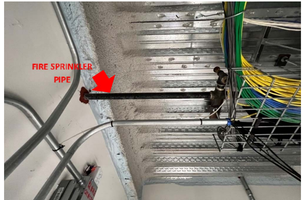
Fire Sprinkler Pipe at Electrical Room (OIG Photo – 10/7/2022)
